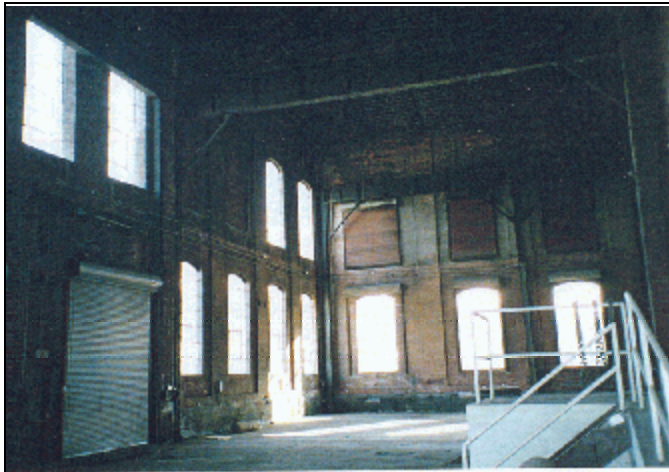
Interior view of the historic Quackenbush Pump House space prior to renovation.
